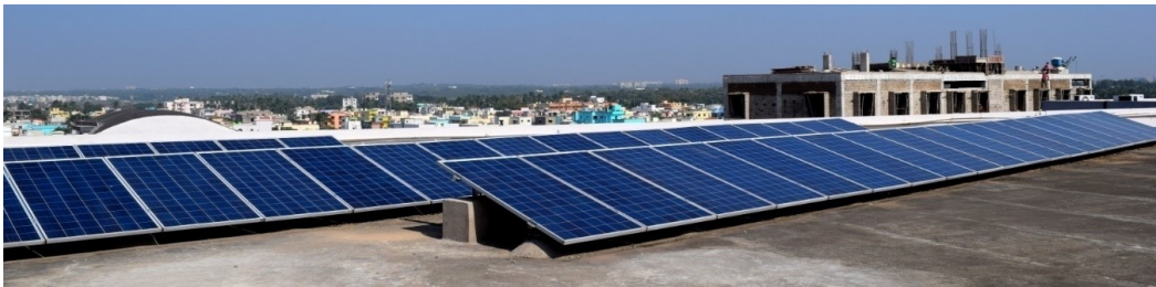
Figure 2: Setup of rooftop-based 11.2 kW PV system at Siksha ‘O’ Anusandhan Bhubaneswar campus.
